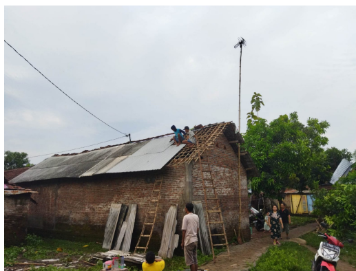
Figure 7. House repairs after the Strong Wind Disaster in Mojowarno District, 2022.
