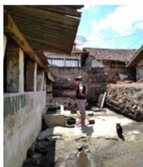
Figure 5. The damaged, clean water supply center
