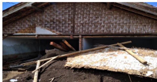
Figure 6. A house buried in sand and abandoned by the owner
