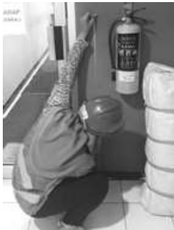
Figure 3. The Height Measurement of Fire Extinguisher at Plastic Sack Industry in 2019
