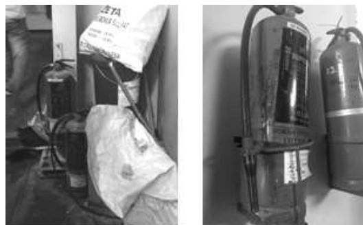
Figure 1. Condition of Fire Extinguisher at Plastic Sack Industry in 2019
