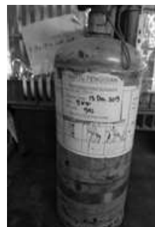
Figure 2. The Condition of Fire Extinguisher Label at Plastic Sack Industry in 2019
