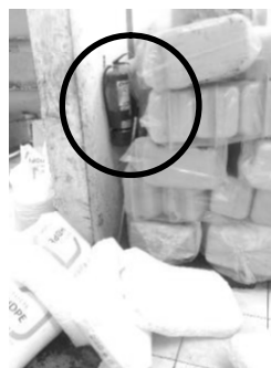
Figure 3. Not Easily Seen and Taken Fire Extinguisher in the Jerry Can Storage Warehouse in September 2019
