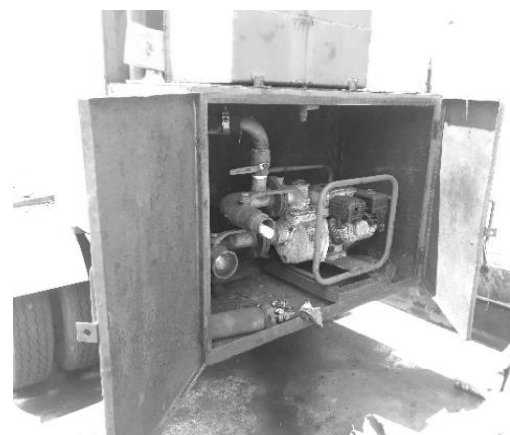
Figure 6. Inappropriate Portable Fire Extinguisher in the Backyard in September 2019
