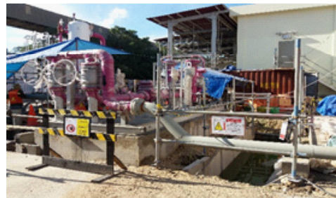
Figure 6. Installation of Symbols and Signs at Amurea II Plant III of Petrochemical Company in 2017
