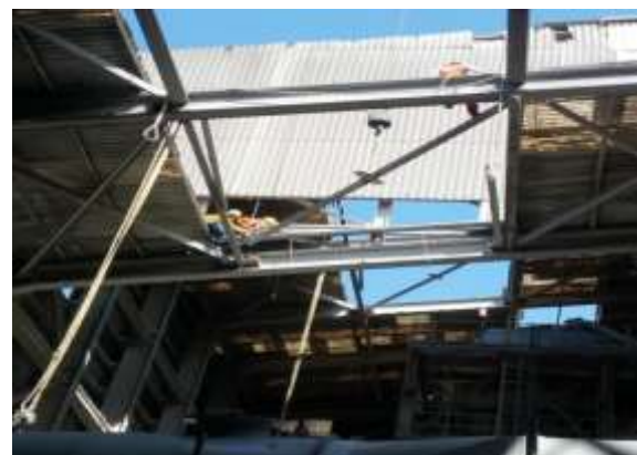
Figure 1. Installation of Bracing on the Roof Cover in a Gresik Fertilizer Company in 2017
