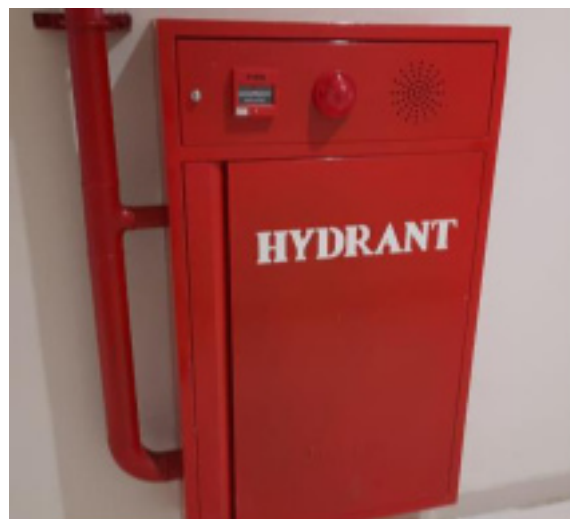
Figure 8. Condition of Fire Hydrants and Alarms in the Chemical Analytics Laboratory of University X Surabaya in August 2020
