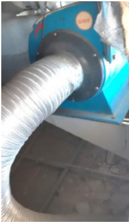
Figure 4. A Fan installed on Hitachi ZA3000 of the Testing Laboratory at the UPT of Occupational Safety Surabaya in 2020
