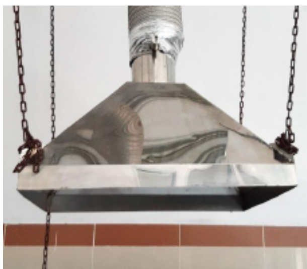
Figure 2. A Hood installed on Hitachi ZA3000 of the Testing Laboratory at the UPT of Occupational Safety Surabaya in 2020
