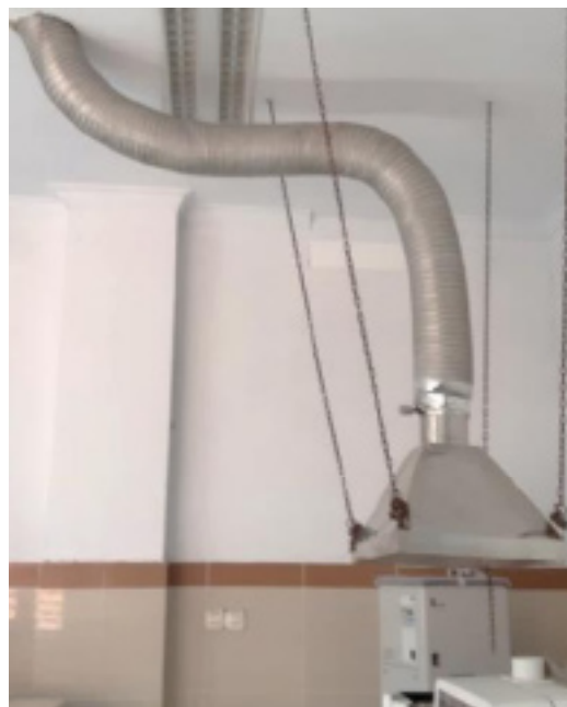
Figure 3. A Duct installed on Hitachi ZA3000 of the Testing Laboratory at the UPT of Occupational Safety Surabaya in 2020
