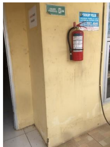
Figure 4. A Fire Extinguisher at Ogan Ilir Police Station
