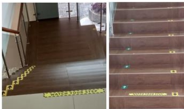
Figure 4. Safety Sign in Main Area
