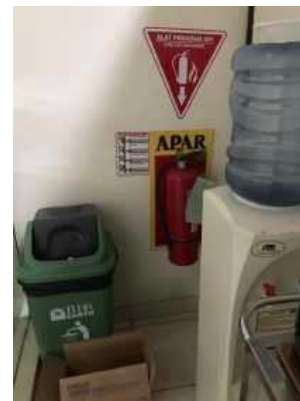
Figure 1. Fire Extinguisher Blocked by Objects
