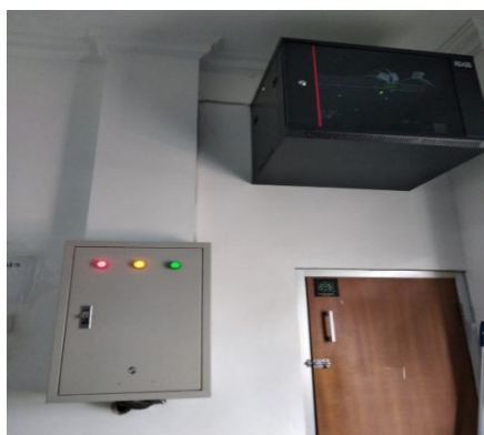
Figure 3. Electrical Control Panel
