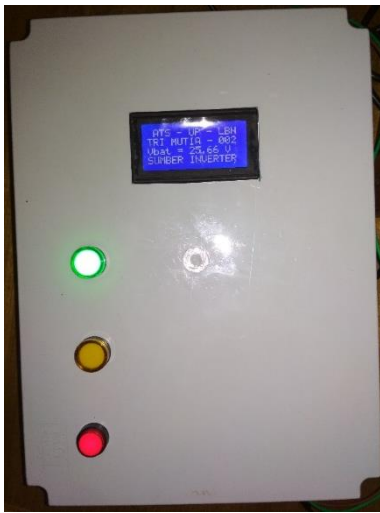
Figure 9 Front view of ATS when battery voltage > 25.5 Volt
