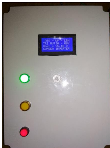
Figure 13 Front view of the panel when the battery voltage is 24.5-25.5 Volts with the rating condition going to undervoltage
