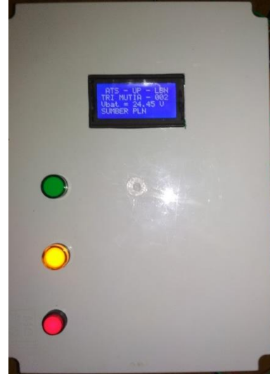
Figure 7 Front view of ATS when battery voltage < 24, 5 Volt
